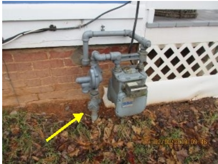
The main gas valve is located at the meter, which is located at the West Exterior.
