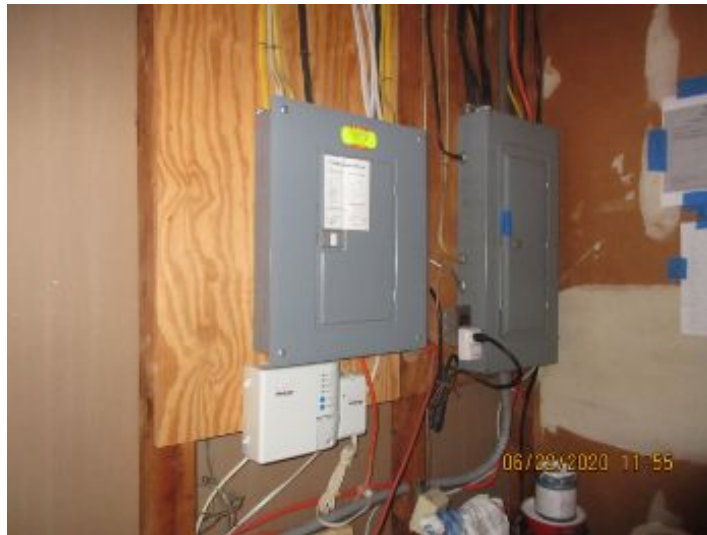
Electrical System Main Service Panel(s)
